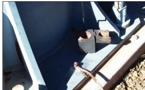
Figure 6a. AWG 2/0 bare copper grounding electrode conductor exothermically welded to a lift tower base. The graphite weld mold can be seen at the upper right of the photograph.
