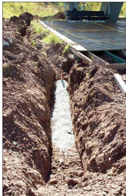
Figure 8b. Overview of one of the chemical electrodes at the lower chairlift terminal station. The electrode is surrounded with bentonite clay to improve electrical continuity with the earth. The ring-ground surrounding the station can be seen at the rear of the scene.
