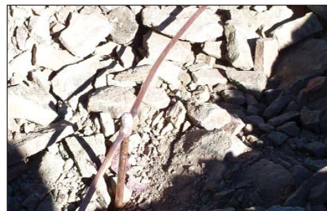
Figure 6b. Grounding electrode conductor exothermically welded to a 5-ft (1.5-m) copper-clad electrode located a few feet from a lift tower. All connections are made using AWG 2/0 bare copper.
