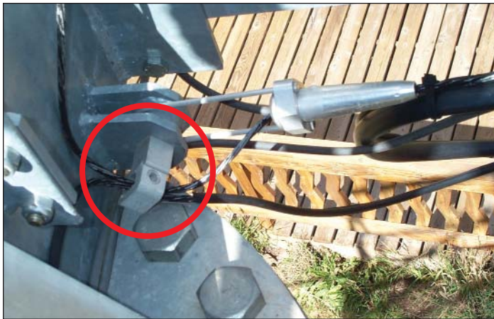
Figure 11. Typical grounding connection between the shield of the chairlift's 50-pair telecommunications cable (black cable, right) and one of the towers. The mechanical setscrew-type connection is seen at the left.
