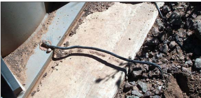
Figure 3. The Chile Express lift's cable support towers were originally grounded with lengths of AWG 1/0 (or smaller). No made electrodes were detected. Although ground resistance was below the 50-ohm limit cited under ANSI B77.1-1999, readings at the 36 towers varied widely. Resulting ground-loop currents were one likely source of the poor power quality that plagued the chairlift's computer control system.
