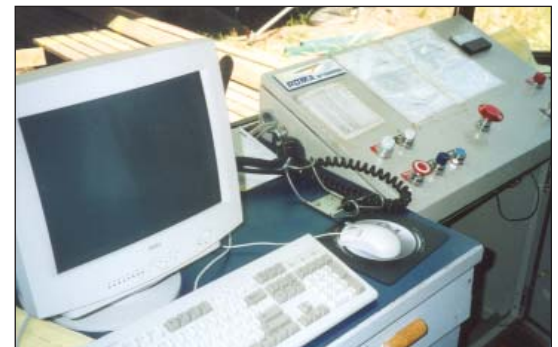
Figure 9b. One of two computers that control the Chile Express chairlift at Angel Fire Ski Resort. For safety, each computer operates on three different types of CPUs.
