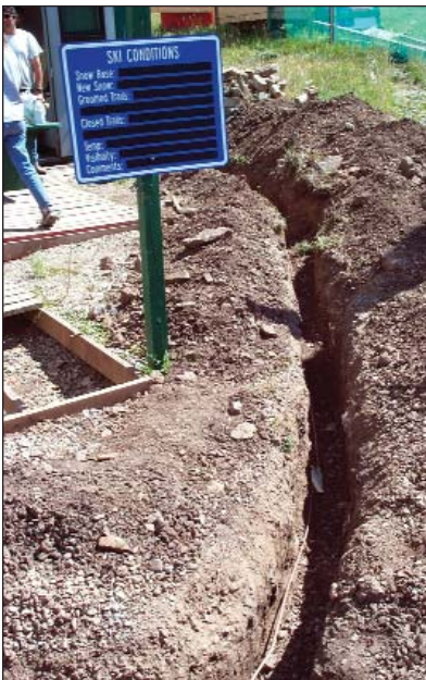
Figure 8a. AWG 2/0 bare copper forming a ring-ground surrounding the Chile Express chairlift's lower terminal station. A similar ring-ground was constructed at the upper terminal station, and both were connected by means of the long copper conductor shown in Figure 7.
