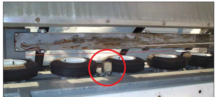
Figure 2b. Dozens of sensors of several types are located along the Chile Express chairlift. The zone sensor shown at the center of this photo checks the position of quad chairs passing through the lift's lower terminal station.
