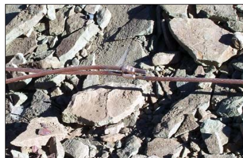
Figure 6c. Exothermic weld between the grounding electrode conductor shown in Figure 9b and a 10,000-ft (3,048-m) length of AWG 2/0 to which all tower grounds were connected.
