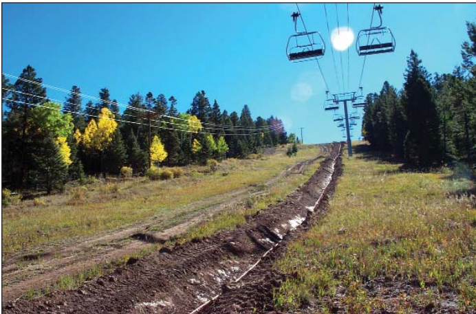
Figure 7. A portion of the 10,000-ft (3,048-m) length of AWG 2/0 bare copper cable connecting all tower grounding electrodes. The cable, visible in the 3-ft (1-m) deep trench, provides a far better electrical connection between the towers than the aluminum messenger wire shown in Figure 5. The low-resistance connection minimizes ground loop currents that formerly plagued the chairlift's control system.
