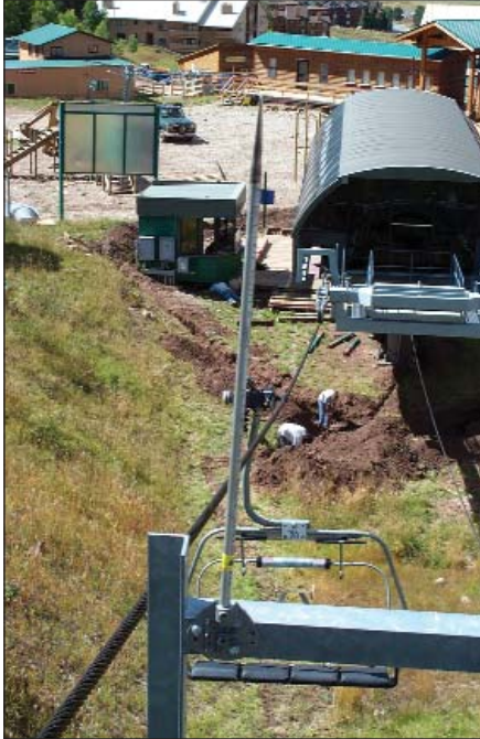
Figure 10. One of six Franklin rods (air terminals) mounted atop each of the Chile Express chairlift's 36 cable support towers. The steel towers themselves serve as down-conductors. A portion of the ring-ground surrounding the chairlift's lower terminal station can be seen in the distance.
