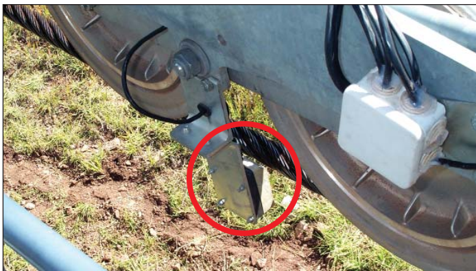
Figure 2c. Proximity sensors (lower center) located on the Chile Express lift's 36 support towers monitor the position of the haul rope with respect to the support sheaves, a potentially life-critical safety factor. Poor power quality and an inadequate grounding system led as many as six of these sensors to fail per day, eventually closing the lift. Cable leads from other sensors on the tower can be seen entering a junction box at upper right.
