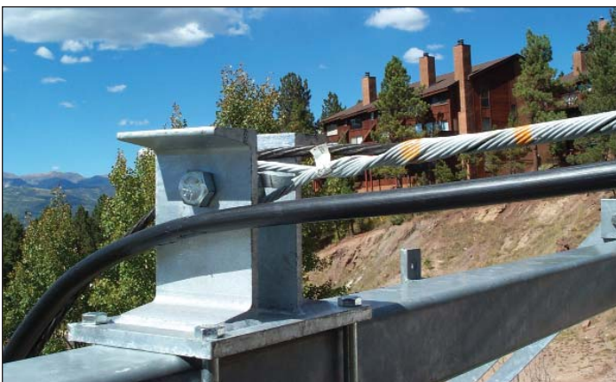
Figure 5. Terminus of the aluminum messenger wire atop a support tower on the Chile Express chairlift. Until extensive modifications were made to the chairlift's grounding system, the messenger wire was the primary electrical connection between 36 individually grounded towers, a situation that helped generate multiple ground loop currents in the system.
