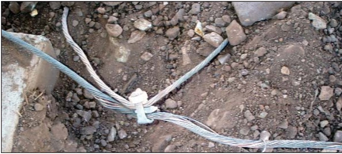
Figure 4. Connections between original grounding electrode conductors at the upper and lower terminal stations were found to be questionable. Some mechanical connectors, while acceptable in many applications, are not recommended for below-grade installations such as this. Corrosion between dissimilar metals, even if only slight, can contribute to high ground resistance values.
